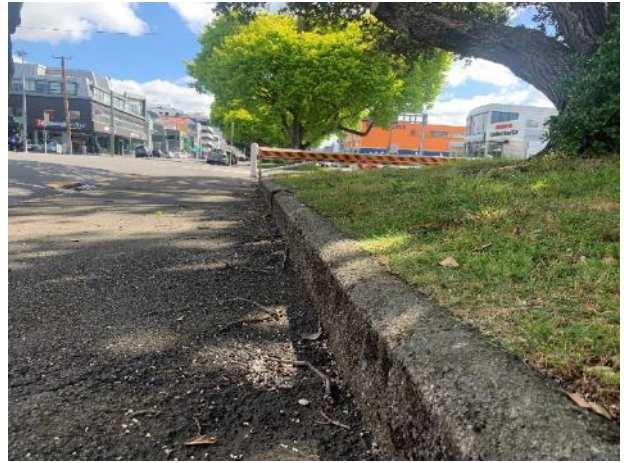
Figure 2-31: Existing footpath lifted by tree roots
